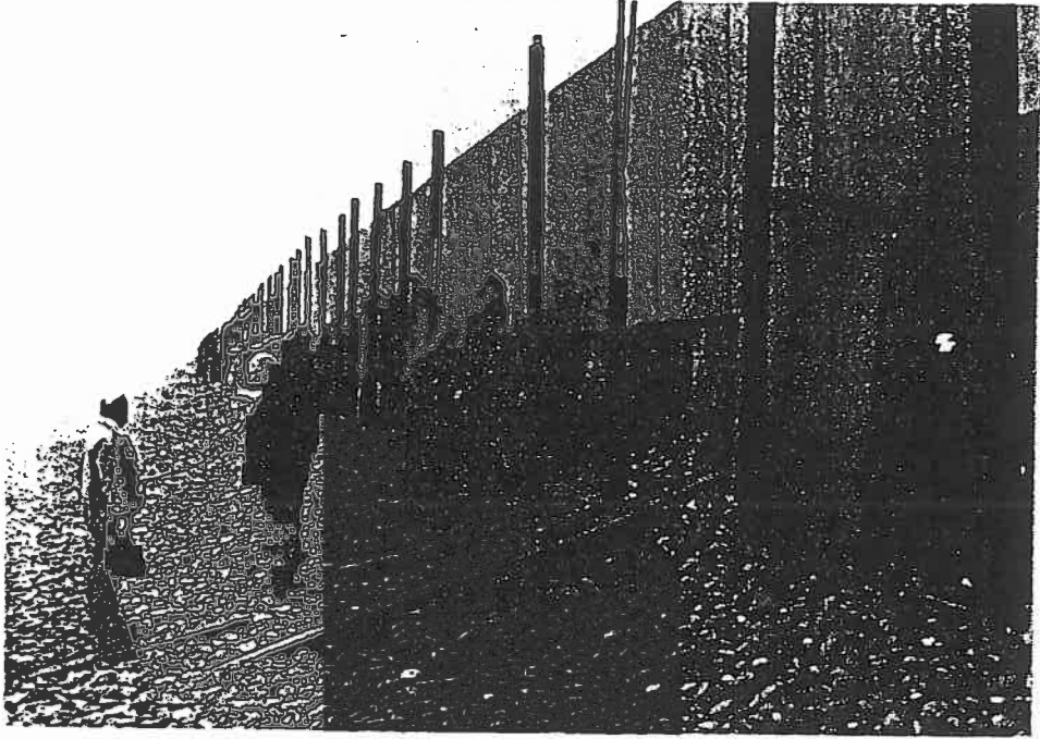
Granity Seawall, October 1988. Note the undercutting of the structure by wave action (Photograph - Don Neale, D.O.C. Hokitika)
